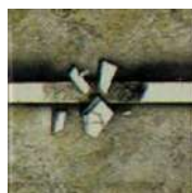
Breached Wall Tile
